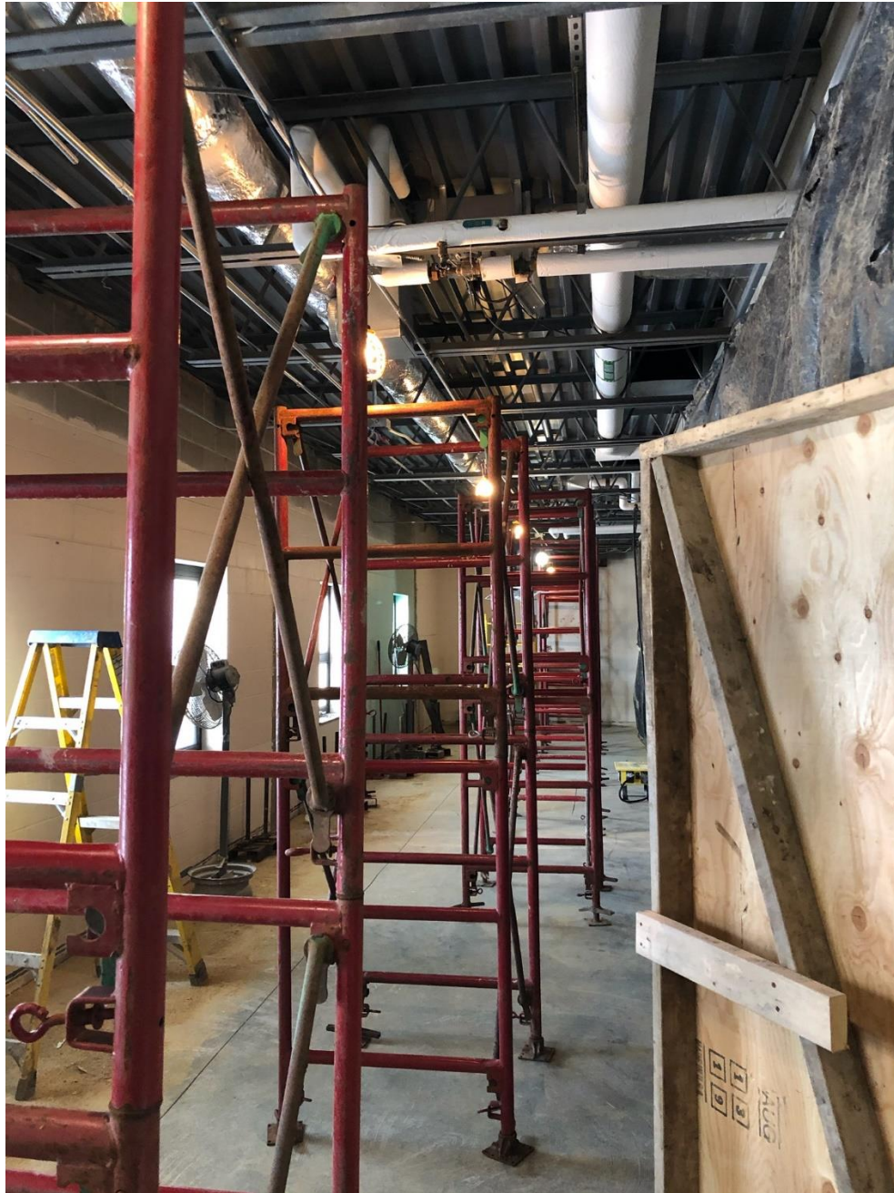
High School/Middle School Additions and Renovations: Demolition and Shoring for wall demolition
