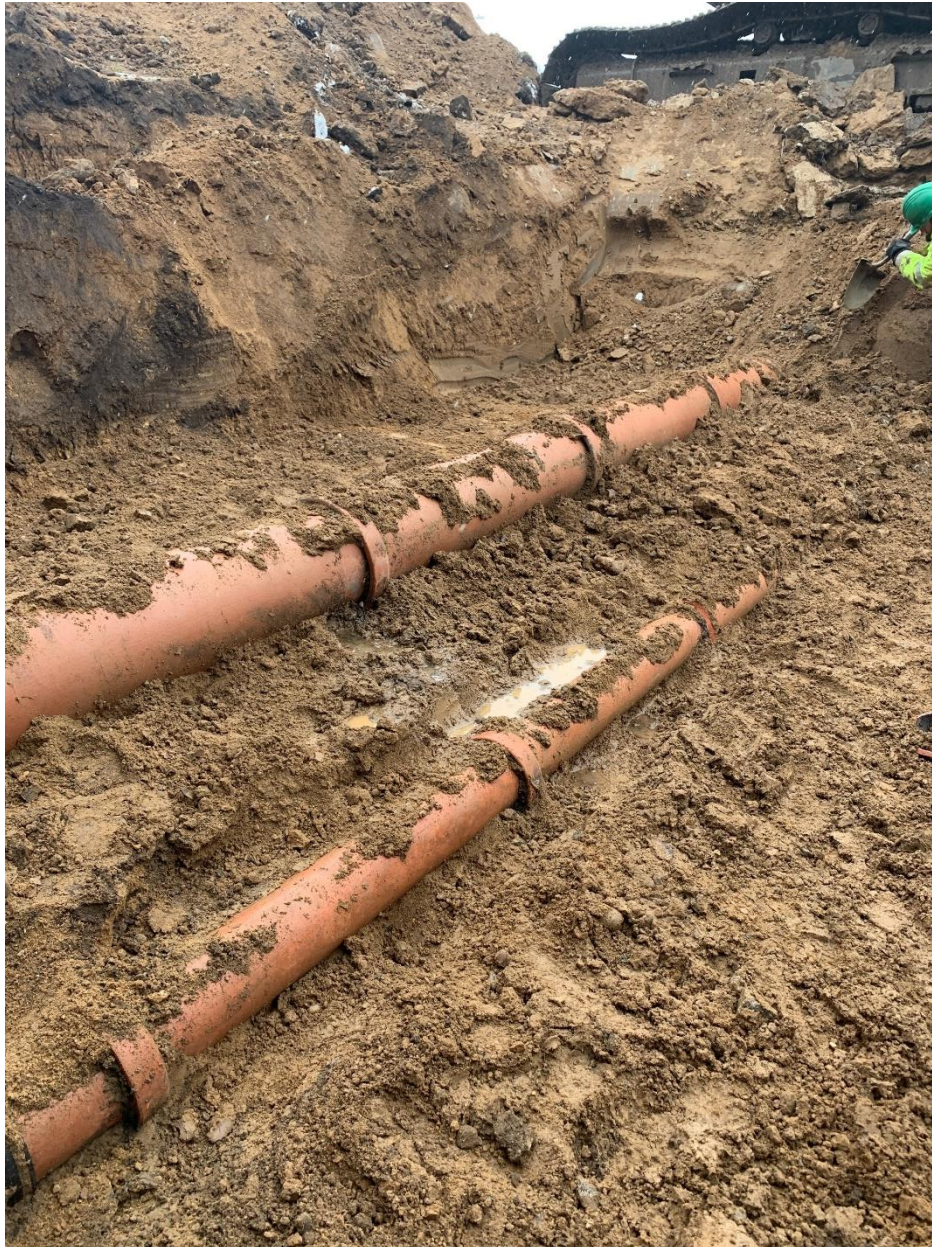
High School/Middle School Additions and Renovations: Excavation and replacement of sanitary and storm sewer
