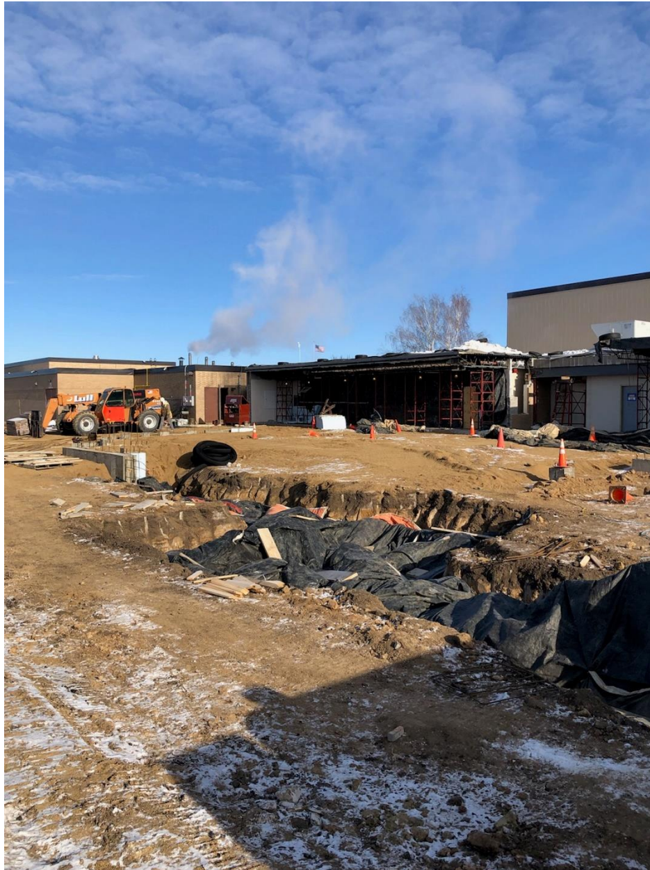
High School/Middle School Commons Addition: Footings and Foundations ongoing, backfill to follow
