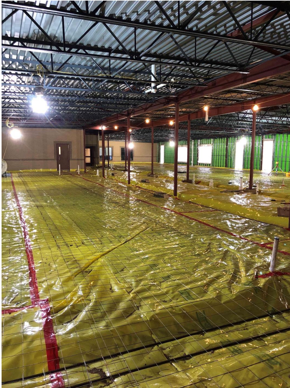
Elementary Classroom Addition Vapor barrier and mesh layed out. Concrete slabs to follow
