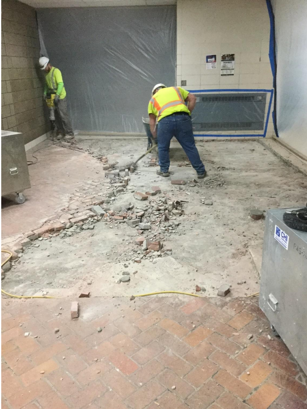
High School/Middle School Commons Addition Demolition of existing brick in corridor, base course to remain. Concrete slab to be poured on top
