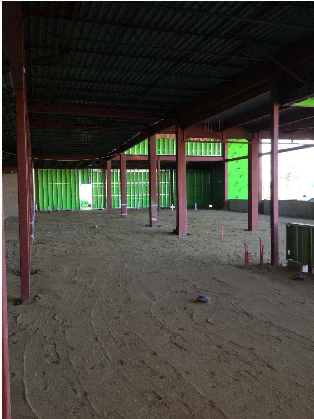
High School/Middle School Commons Addition: Grading complete, vapor barrier and wire mesh installed Thursday/today
