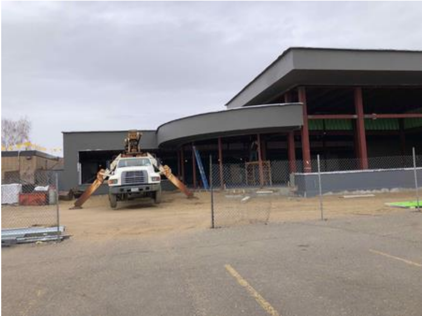
High School/Middle School Commons Addition: Exterior air barrier applied. Brick and parapet flashing to follow.
