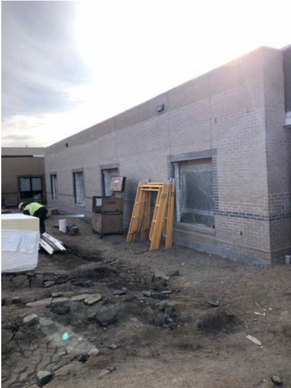
High School/Middle School Commons Addition: Exterior air brick completed on parking lot side
