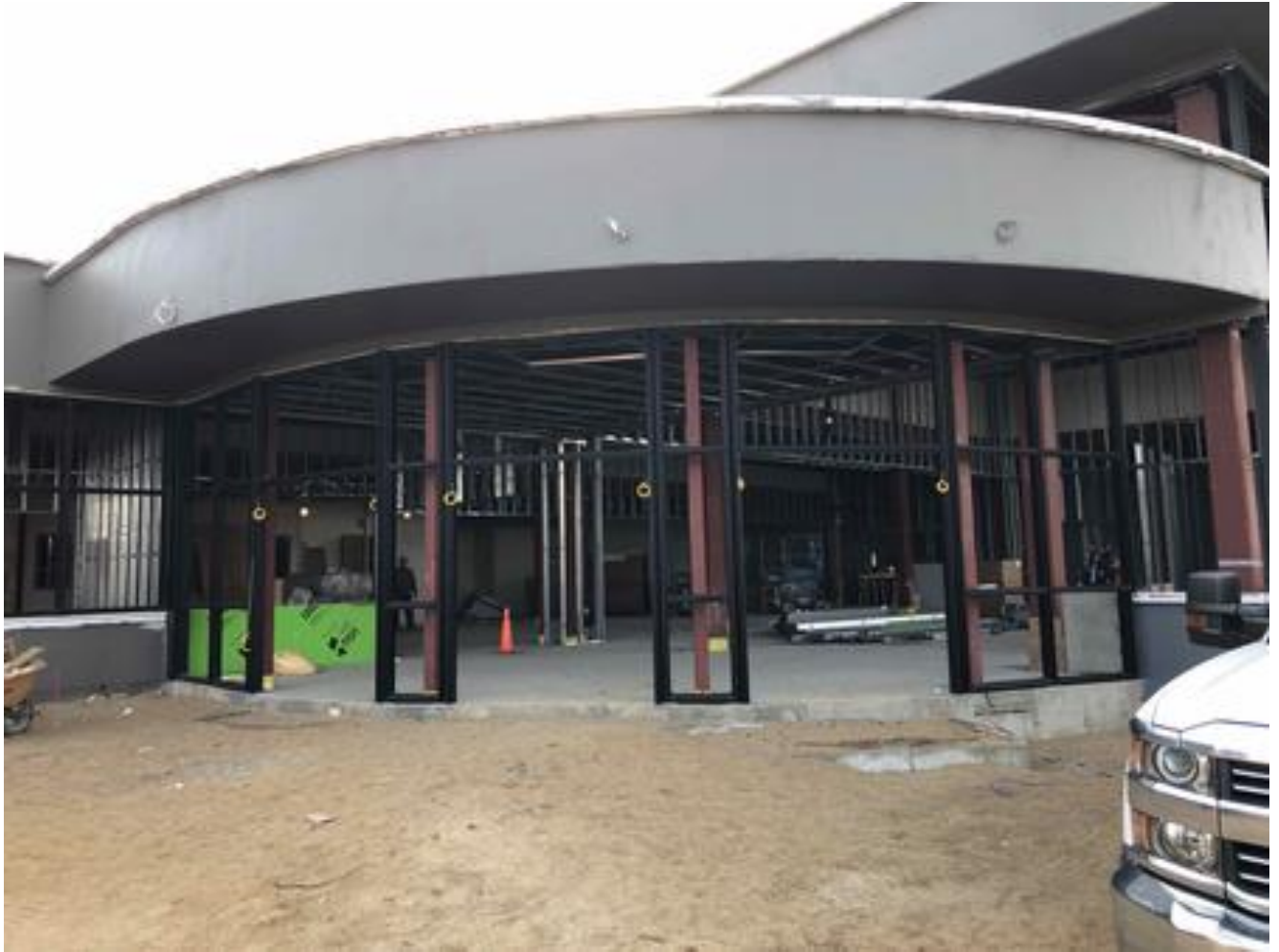
High School/Middle School Commons Addition: Window frames installed at office windows, front entry and curtain wall
