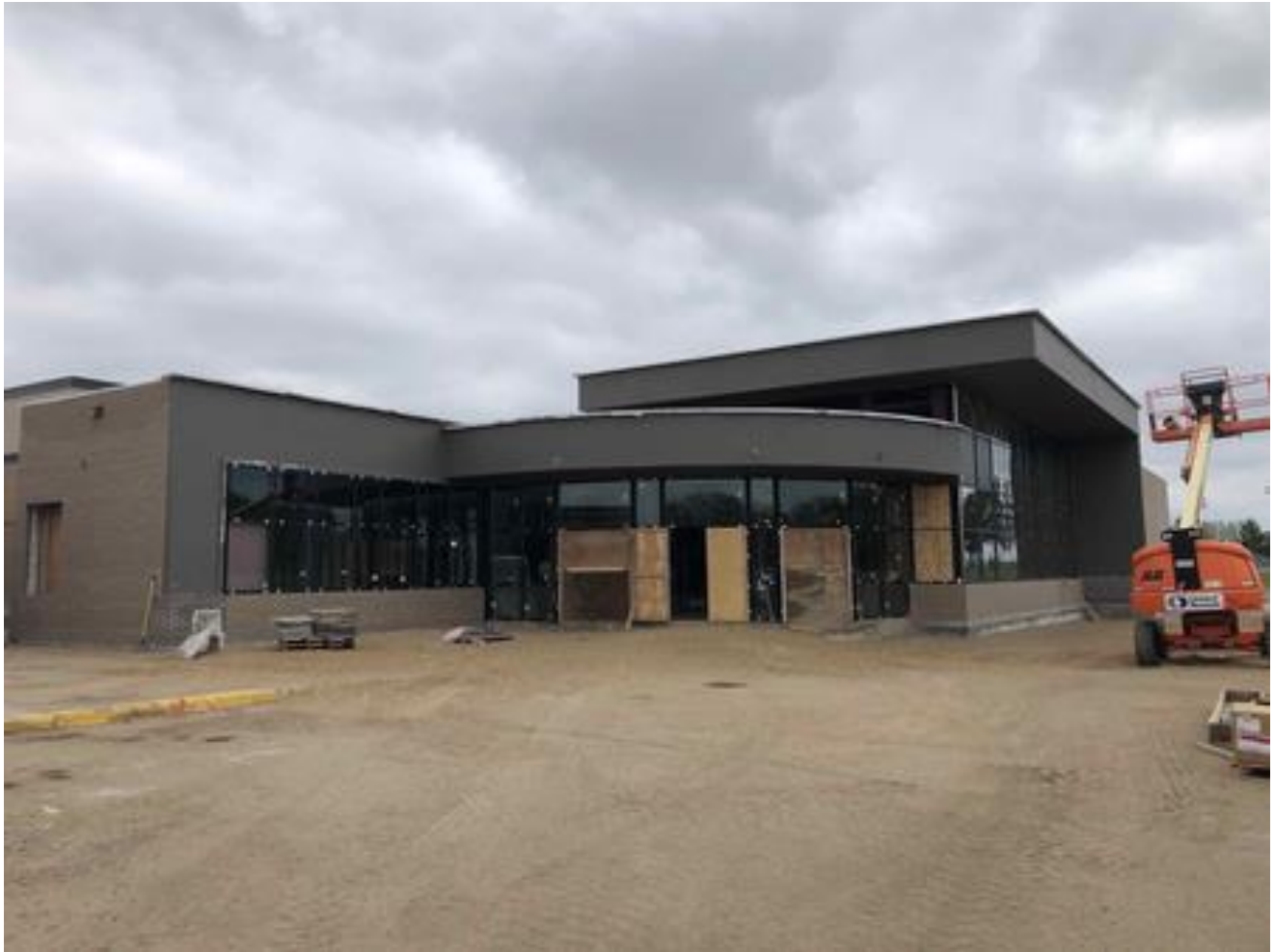
High School/Middle School Commons Addition: Glazing installed, brick almost complete. Metal panels to follow
