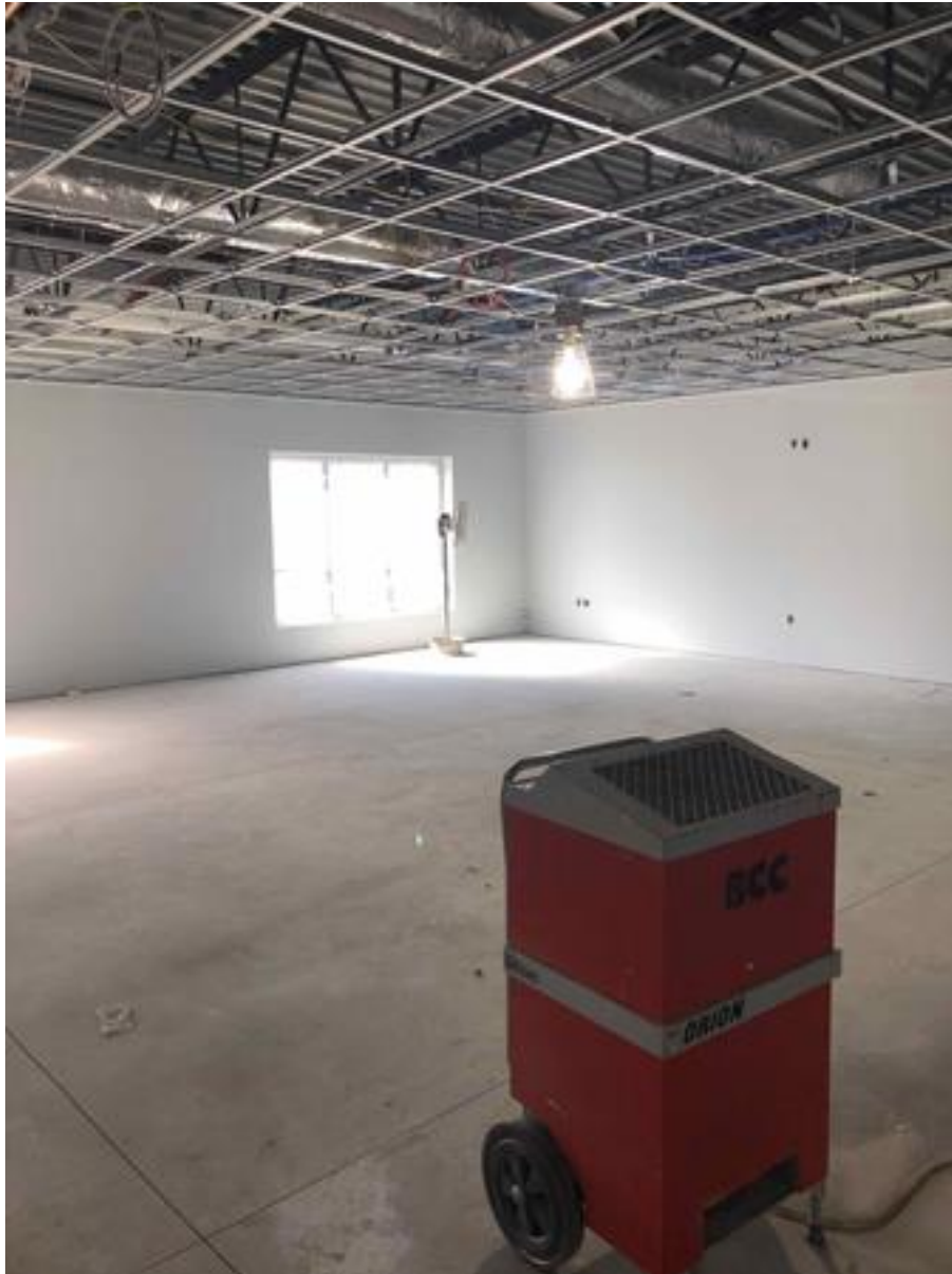
Elementary Classroom Addition: Painting an grid complete, casework and tile to follow
