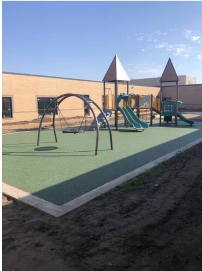
Elementary Classroom Courtyard: Playground equipment and poured in place complete. Engineered wood fiber to follow
