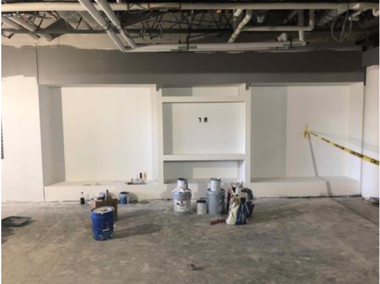
High School/Middle School Commons Addition: Display case framed and painted, casework installation to follow
