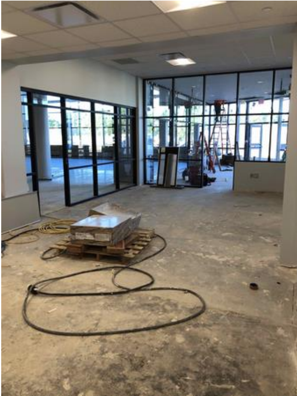
High School/Middle School Commons Addition: Offices painted. Windows and frames installation. Doors and flooring to follow
